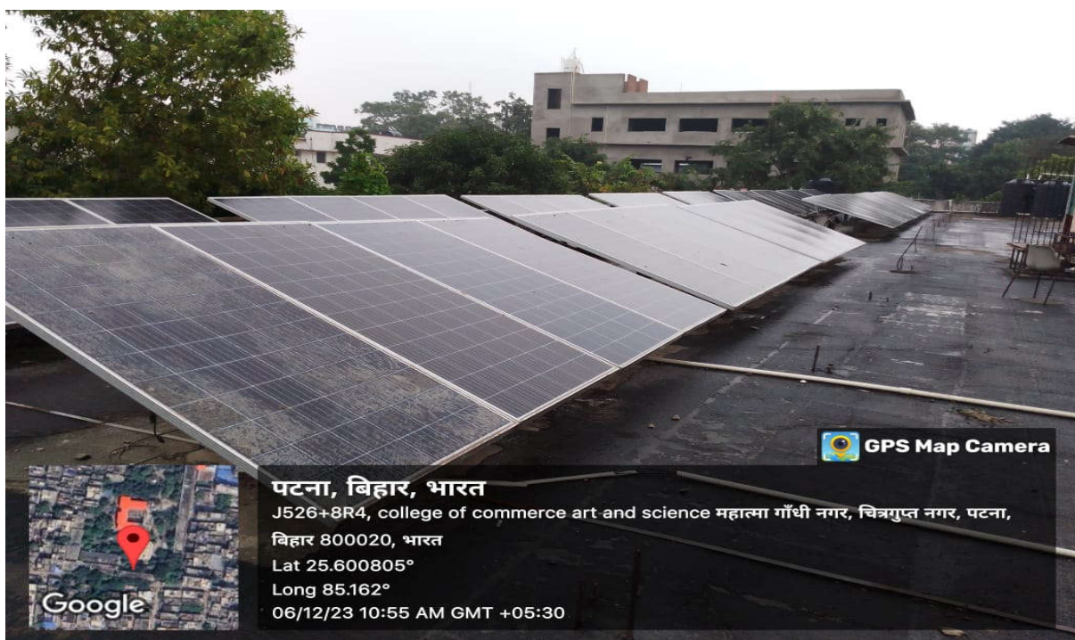
Fig.: Solar Panels installed in the campus
